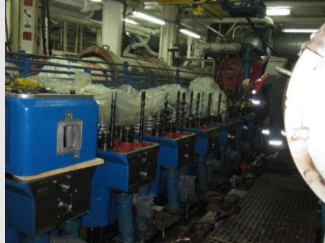
Engine conversion to dual fuel
