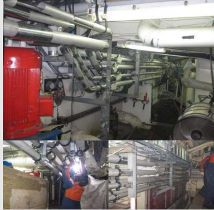
High pressure pipes
